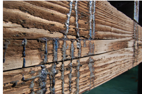
Online Case Study 6 Figure A Creosote-treated timber left to dry in treatment yards drip creosote and lead to contaminated soils and groundwater.
